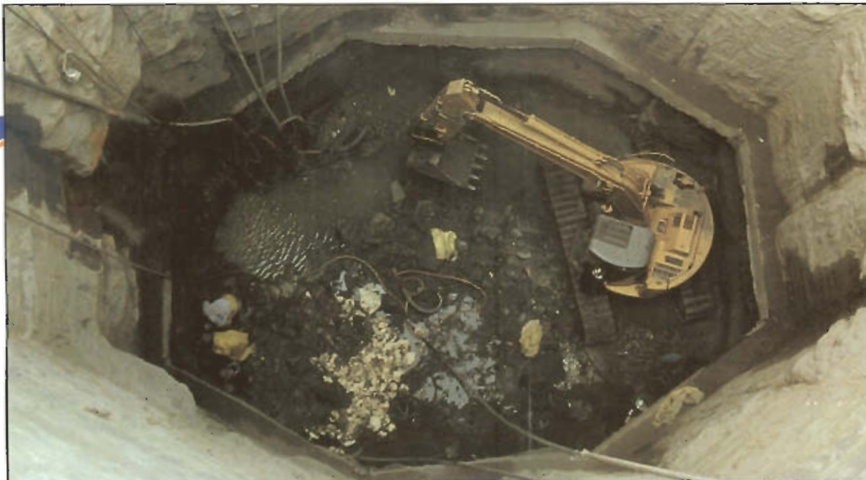
As part of a recent tunnel project in Weymouth, a Mattuchio operator works 80 feet below the surface with a Komatsu PC228US tight-tail-swing excavator.
