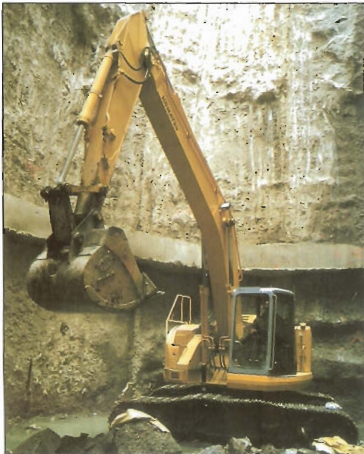
The operator on this Komatsu PC228US excavator from C.N. Wood in Burlington uses the bucket as well as a Kent KQT22F hammer, also from C.N. Wood, on the Weymouth tunnel project. By the end of the job, the shaft will be 30 x 40 x 240 feet deep.
